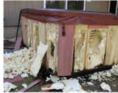
Leaks are the hardest thing to find in a full foam hot tub.
